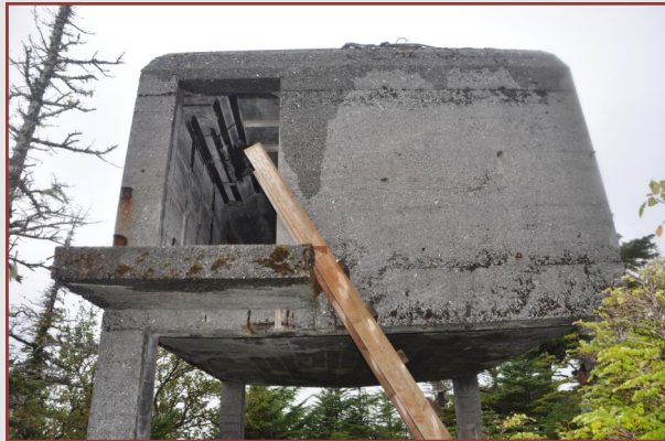
Base end station on Ataku Island
