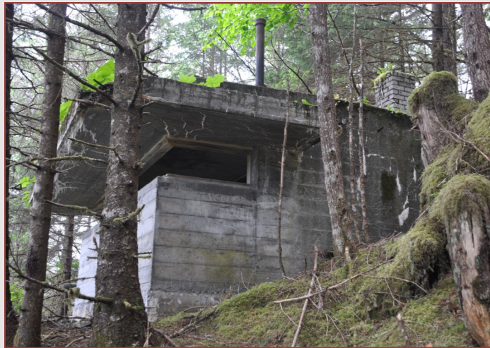
Distant Electric Control (DEC) station, Sound Island
