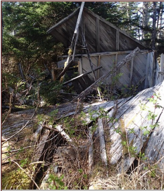
Collapsed Mess Hall, Little Biorka Island (USACE, 2014)
