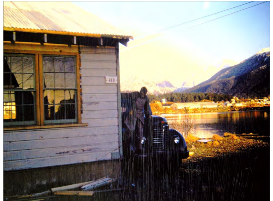
Mt. Edgecumbe Students finishing a home on Charcoal Island circa 1950s (G. Nelson photograph)
